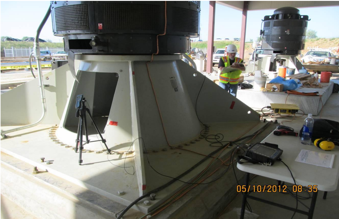
Pump and Motor #9 monitoring equipment and data collection
