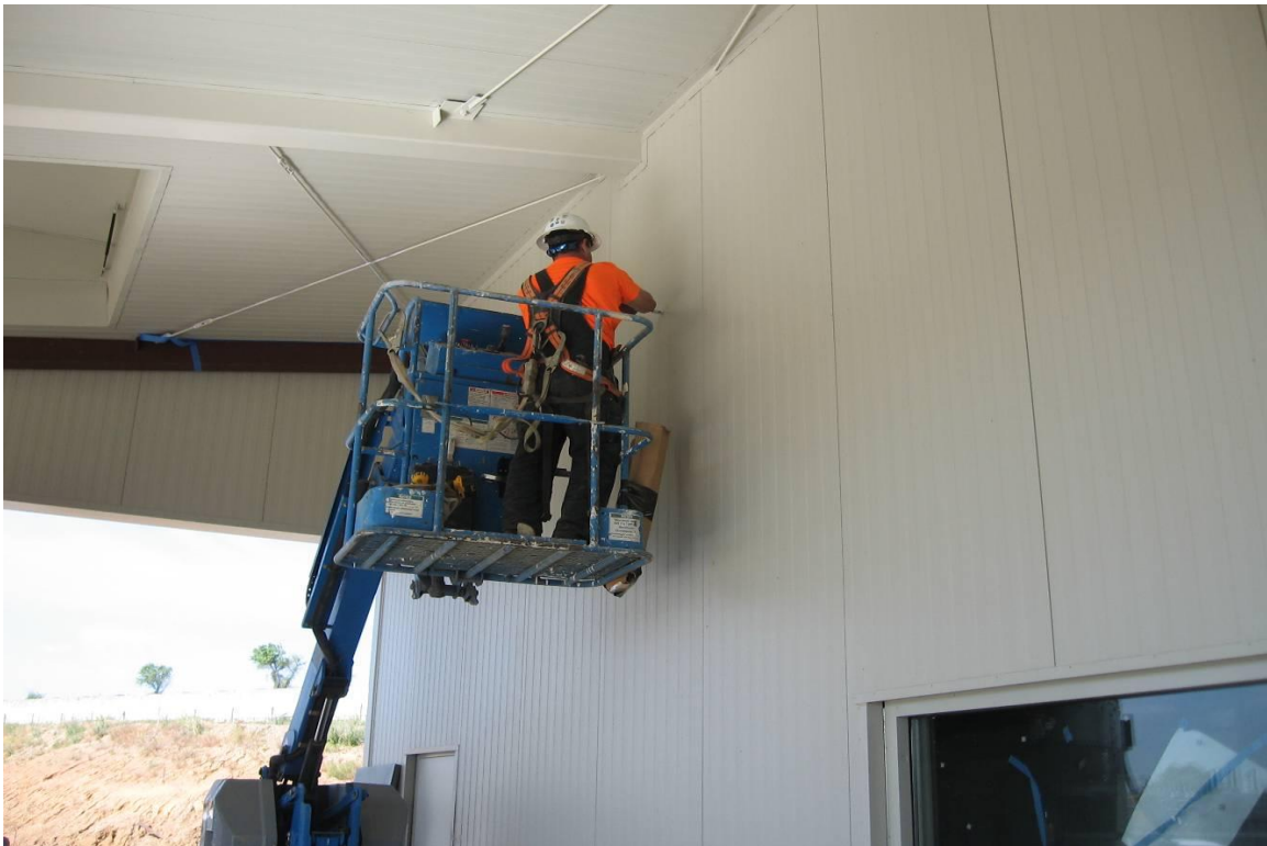
Subcontractor Central Sierra drilling holes for the exterior lights on the downstream side of the control building.
