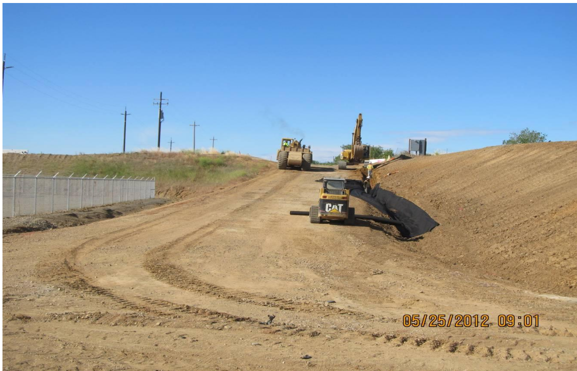
Subcontractor Meyers Earth Work constructing drainage ditch along the switchyard access road
