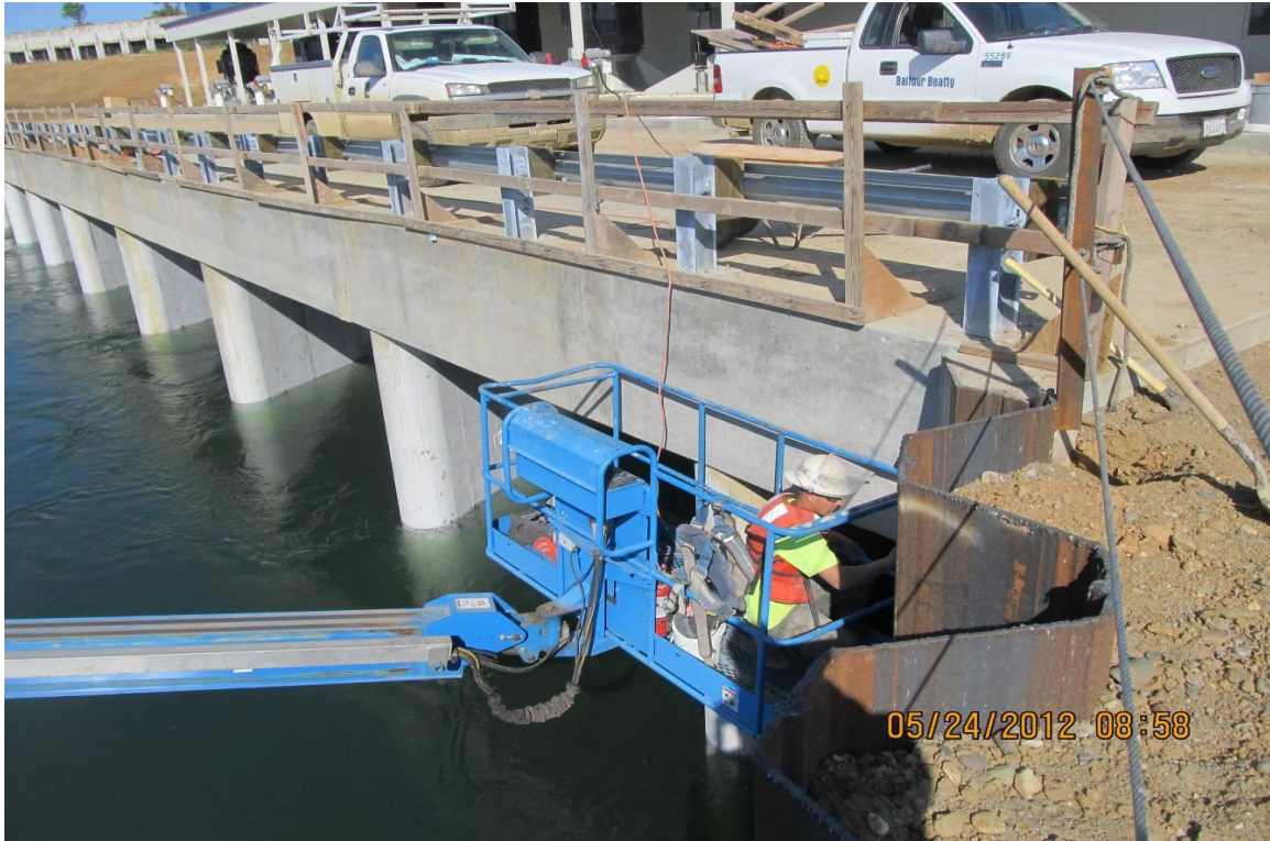
Balfour Beatty laborer making concrete repairs at the afterbay wall and canal transition sheet pile wall.
