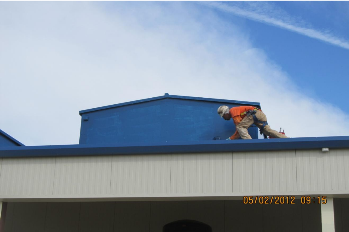
Subcontractor FD Thomas coating the roof hatches to match building roof color
